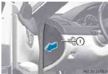
Fuse box on driver's side
